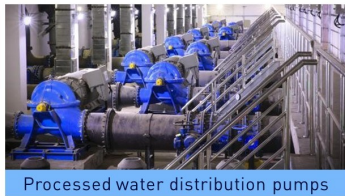
Processed water distribution pumps
